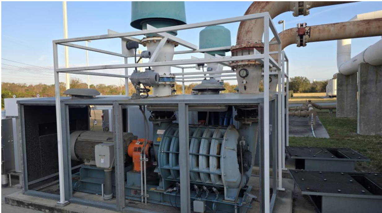
Photo of Centrifugal Blower
